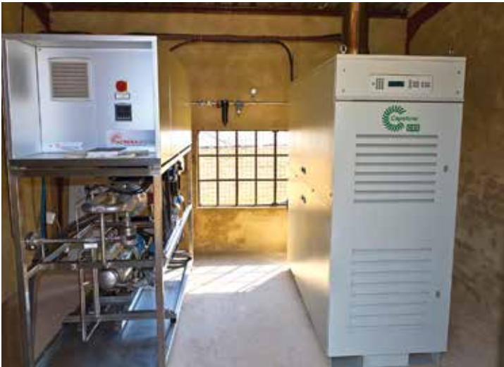
A digester gas-fueled Capstone CR65 microturbine provides power to Swineline Farm in South Africa.
