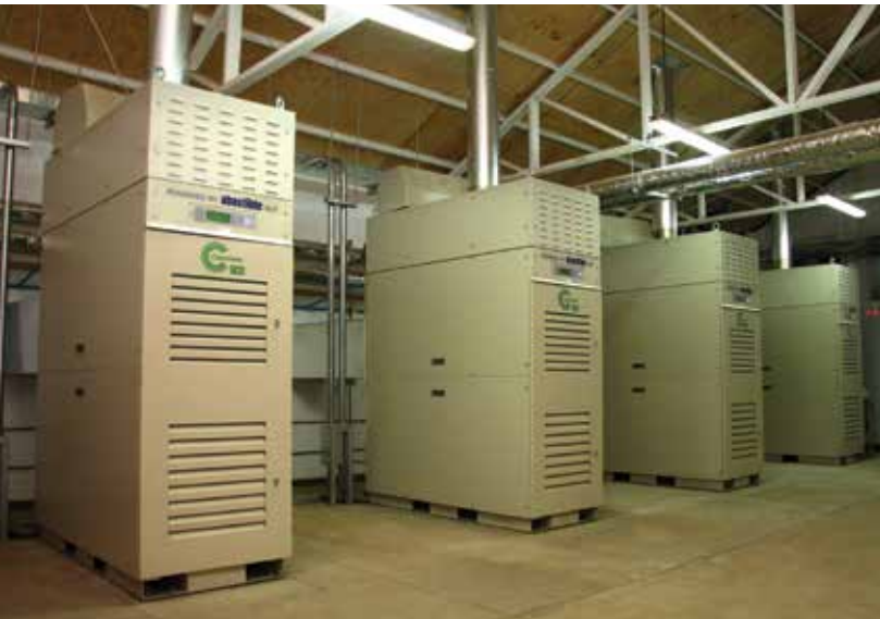
The cogeneration system supports 100 percent of power demand for this luxury hotel and is capable of delivering 1,752GWh of electricity and 3,504GWh of thermal energy per year at full load.
