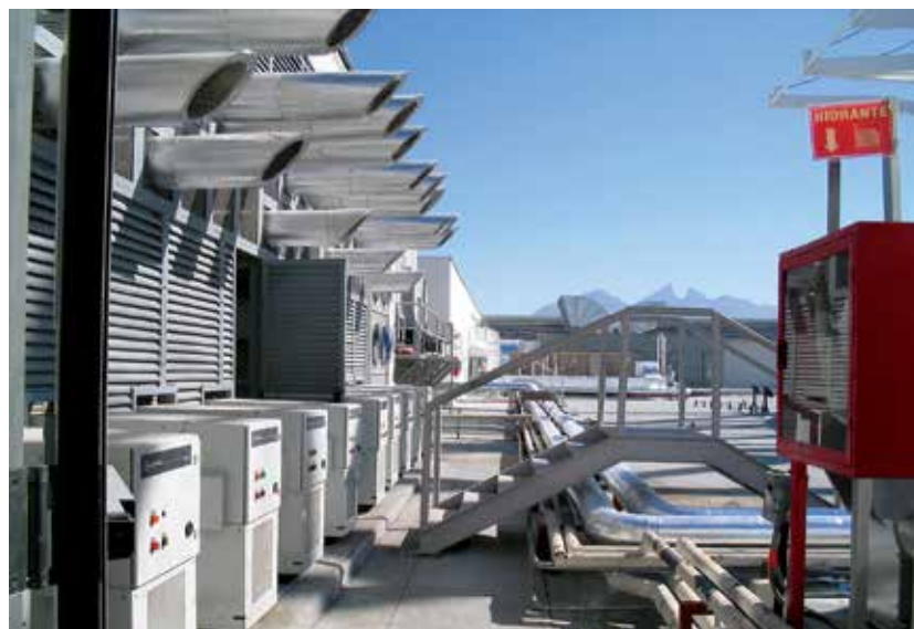
Twenty Capstone C65 microturbines produce 40 percent of the electrical power needed to operate a department store in Monterrey, Mexico.
